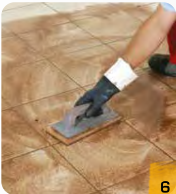
6 Level the surface using wet soft felt pad, cleaning it frequently with a good amount of water.
